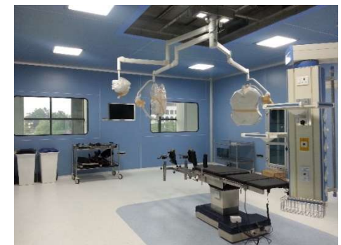
Facility with the company's clean panels installed (walls, ceilings, windows, doors, etc.)
