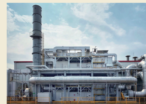
RTO for new B line
