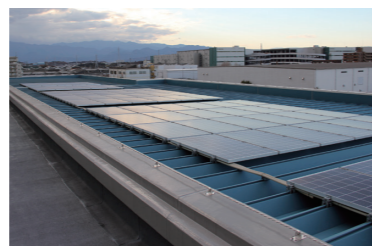
Solar panels installed on the rooftop
