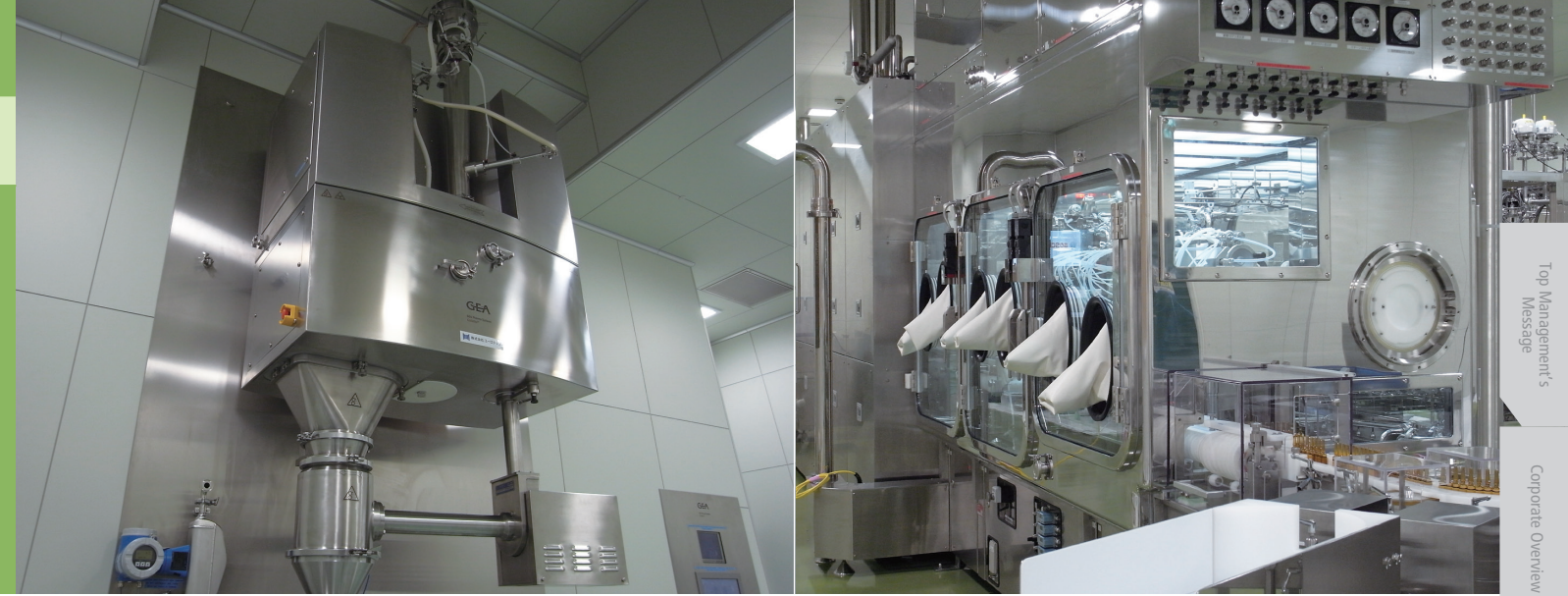
Manufacturing equipment compliant with the containment of high-activity preparations
